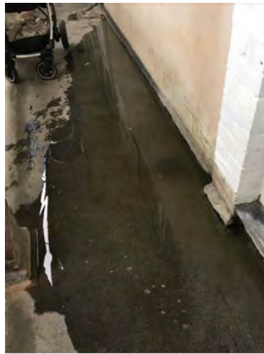
Figure 6.6: Flooding in the external galleries of the maisonette blocks.
