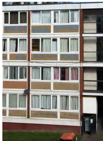
Figure 6.7: Façade showing the panel below the windows, the slabs and parts of the façades that need to be repainted.
