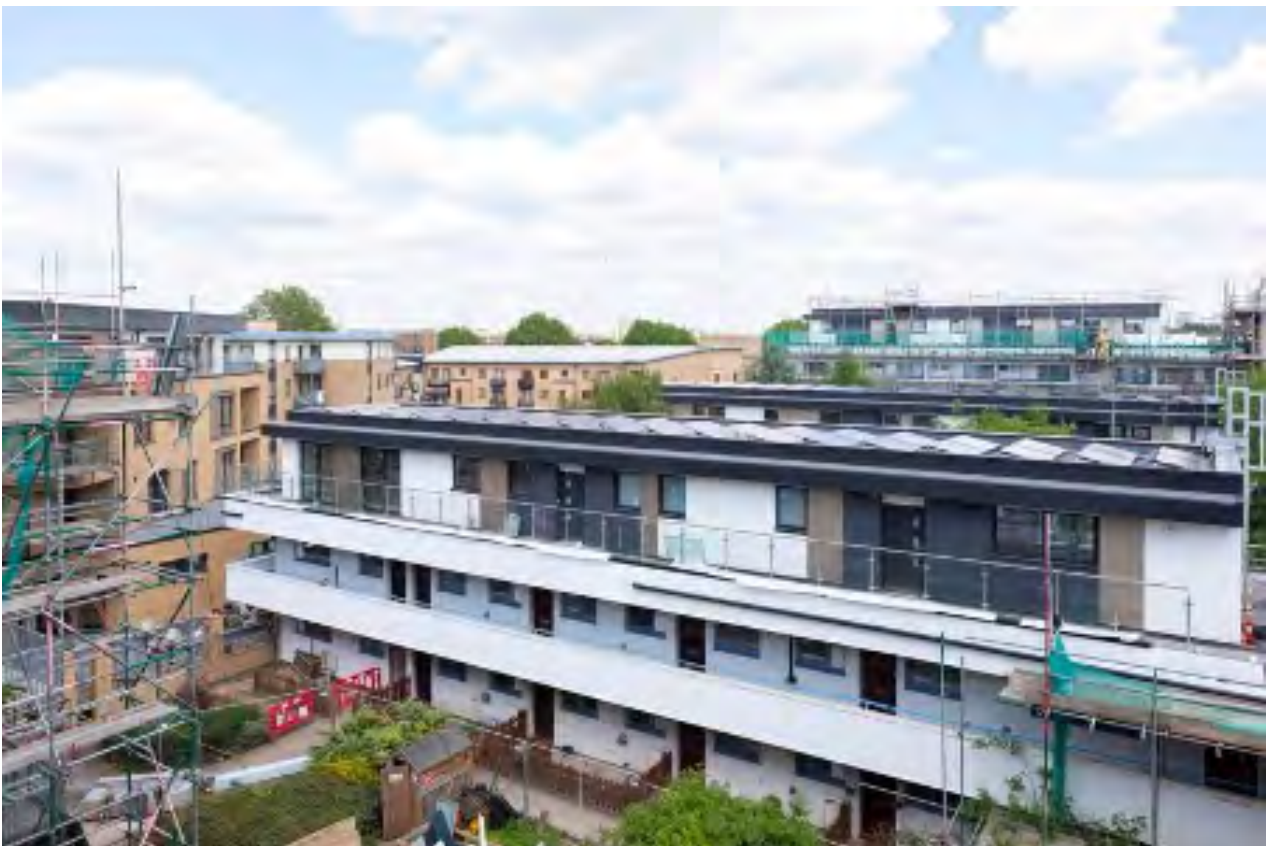
Figure 6.10: Walerton and Elgin Community Homes, community-led scheme that builds new social rent homes through roof extensions, which also include the installation of solar panels.
